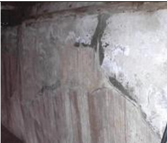
Foundation wall with inward movement.
