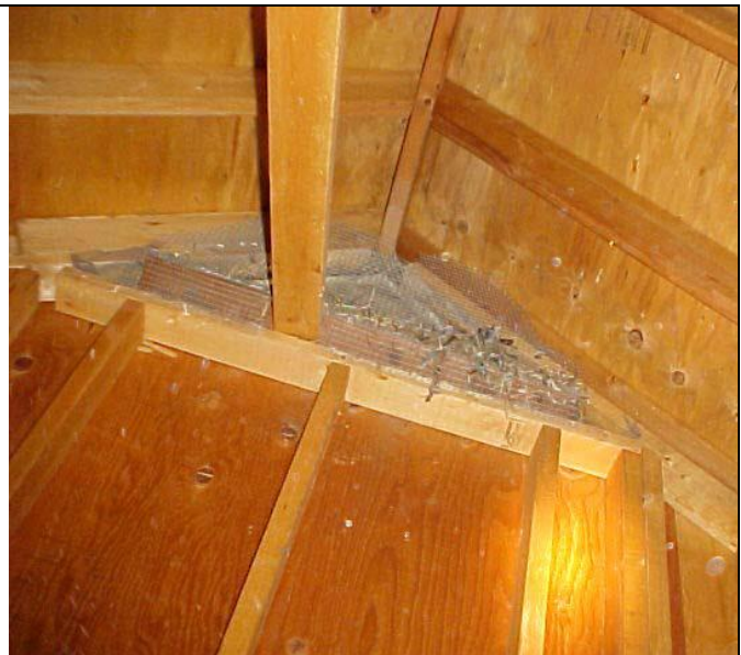
Even if there is an interior screen birds will sometimes build a nest within the louvres if there is enough room. In this case it may be necessary to install the wire mesh on the outside of the gable vent.
