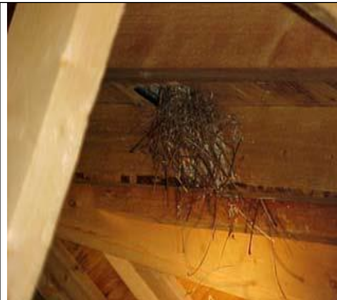
This is a nest that was built in a roof vent. I have seen entry locations through eaves and other small holes in the siding of a home.
