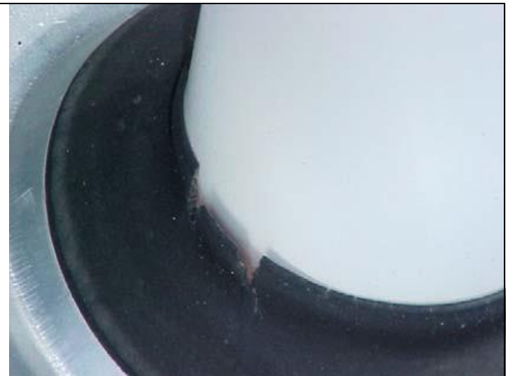
Close up view of a damaged roof boot.
