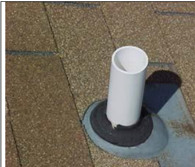
This photo shows a typical sewer gas vent pipe with a deteriorating boot.
